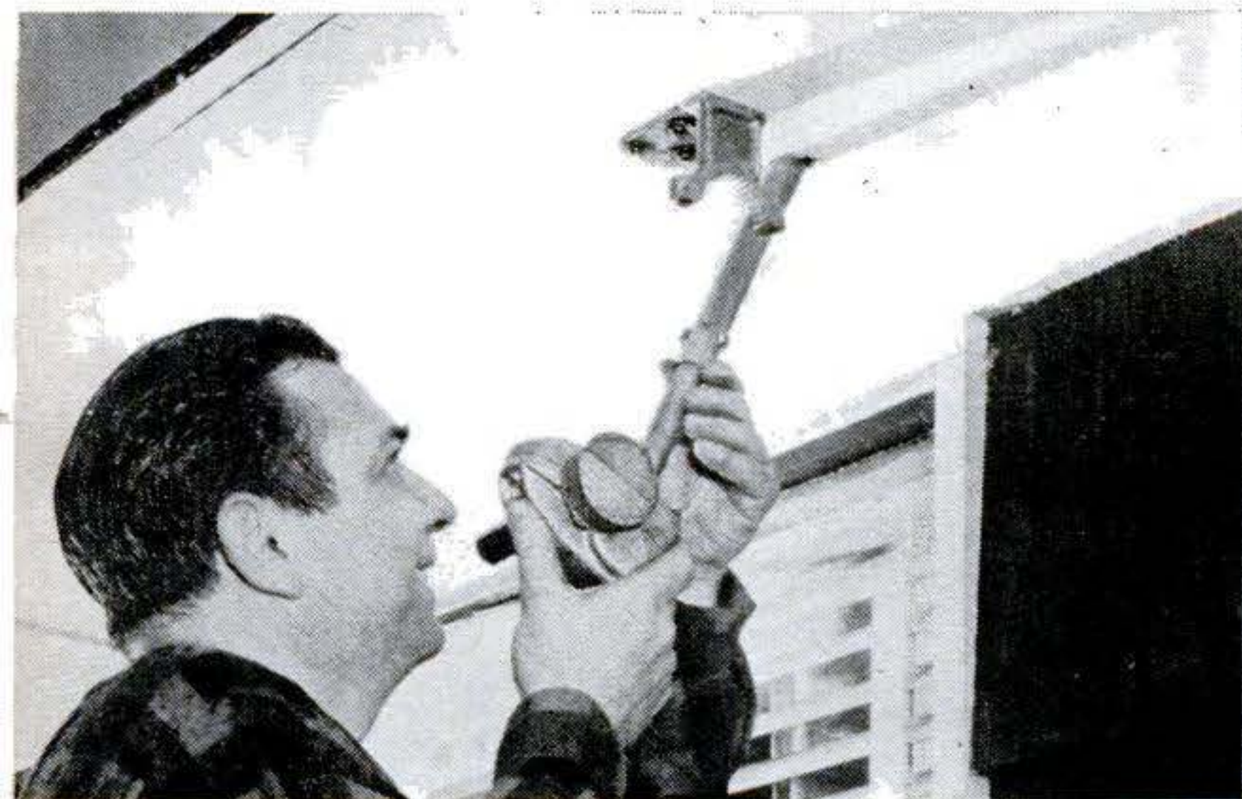
SHAFT HOLE WAS SPOTTED by sighting along mounting bracket and gear-case collar. An extension shaft of light aluminum tubing was bolted on and pushed through into the attic.
